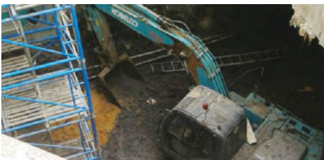
Excavation for Entrance-C (Roof to Concourse) work in progress at Kilpauk Metro Station
